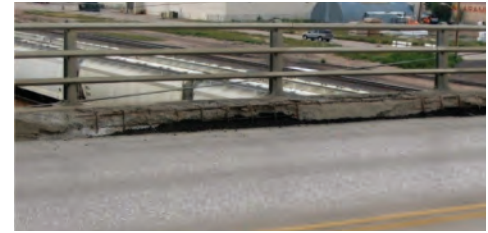
Chips on Front Side of Curb with Exposed and Corroded Reinforcing Steel
