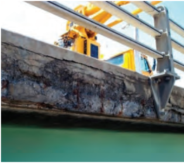
Clark Street Viaduct Curb with Exposed and Corroded Reinforcing Steel (Photo: Courtesy of WYDOT)
