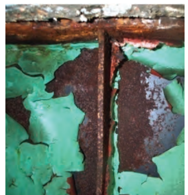
Falling Paint System with Pack Rust at Top Figure
