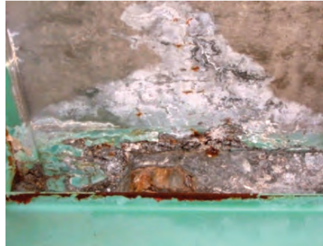
Chips, Delaminations, and Rust Staining on Underside of Deck
