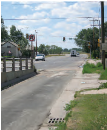
Service Road Transitioning to Turn Lane (Looking West) Clark Street East of Cedar Street
