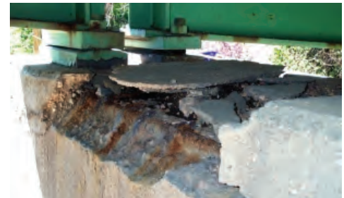
Severe Chipping with Loss of Concrete Corroding Reinforcing Steel between Bearings
