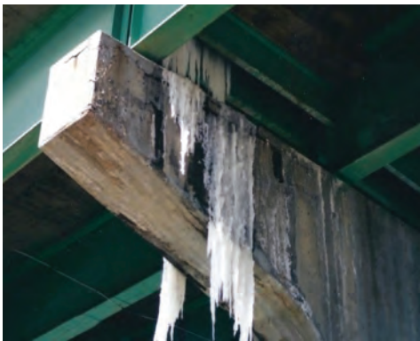
Evidence of Joint Failure Over Pier
