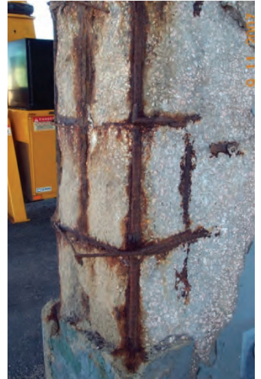
Clark Street Viaduct Pier with Corroded Concrete and Reinforcing Steel (Photo: Courtesy of WYDOT)
