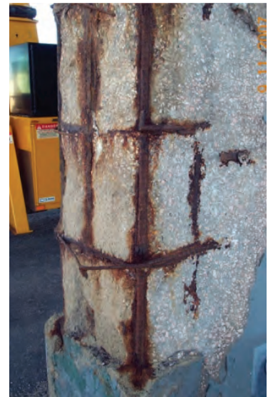
Clark Street Viaduct Pier with Corroded Concrete and Reinforcing Steel (Photo: Courtesy of WYDOT)
