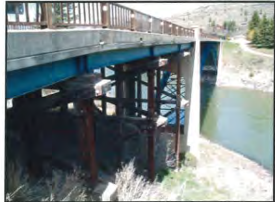
Wooden support structure installed due to an active landslide at Snake River bridge (MP 141.08).
