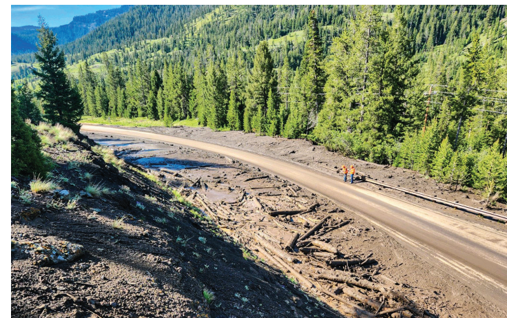
Basin Maintenance Foreman Scott Thomas uses an excavator to move mud and debris from a plugged box culvert. The box culvert became blocked as mud and debris rushed down the mountain on the northside of US 14/16/20. Thomas was able to get the box culvert reopened.
